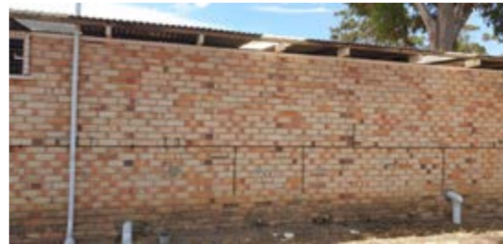
Deterioration of single leaf brickwork to height of 450mm AGL to whole length of southern elevation will require works to rectify.
