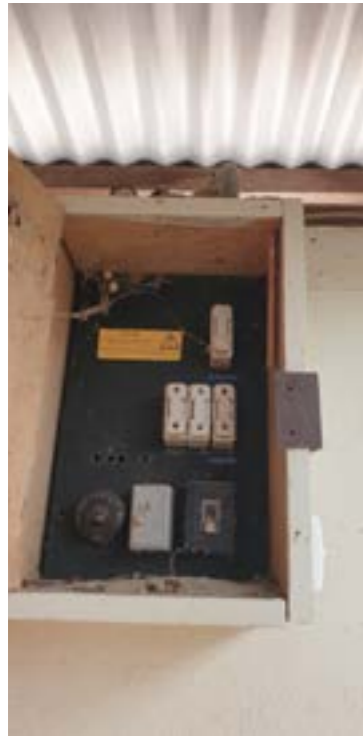
Existing services should be assessed for compliance and capacity to ensure risk minimisation and functionality to cope with future (increased) useage requirements
