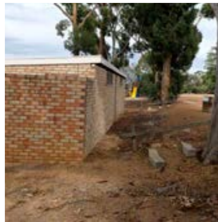
Figure 8 Existing Ablution limited access
