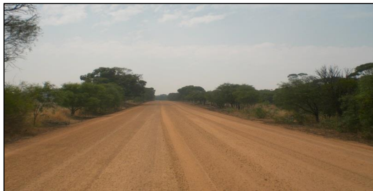
From slk 18.650 highlighting the loose and dusty road surface and the need for the reduction of the vegetation re growth
