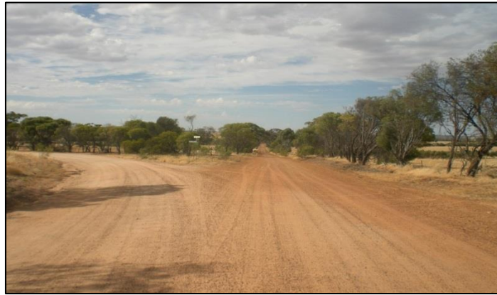
From Malyalling road looking south highlighting the angle of the Y junction
