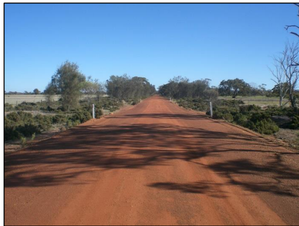
At slk 14.44 looking west through number two and three flood ways highlighting the typical narrow road design
