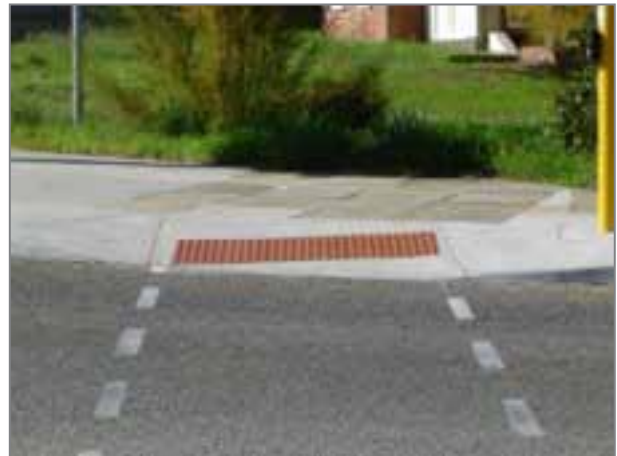
Incorrect Camber: Corner of Aberdare Road and Railway Parade, Nedlands
